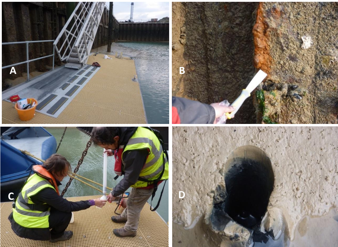
Figure SH2: Images of Shoreham Harbour environment and corrosion. (A) Study site at the Dredger Berth, surrounded by steel pile wall. (B) Corrosion sampling from floating pontoon. (C) Water sampling from floating pontoon. (D) Site of sediment core retrieval.
