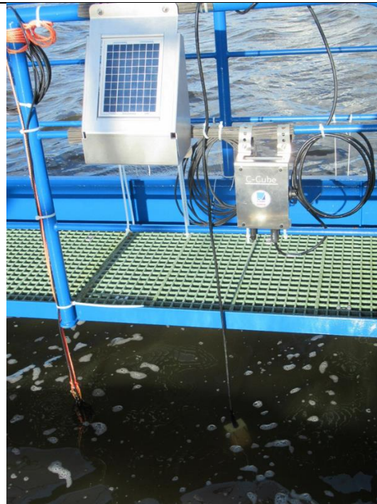
Figure 14. Installation of the corrosion sensor with solar panel at the raft exposure site.
