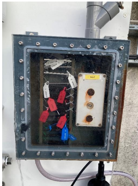
Figure 7. Coupon box at the BASF demonstrators
