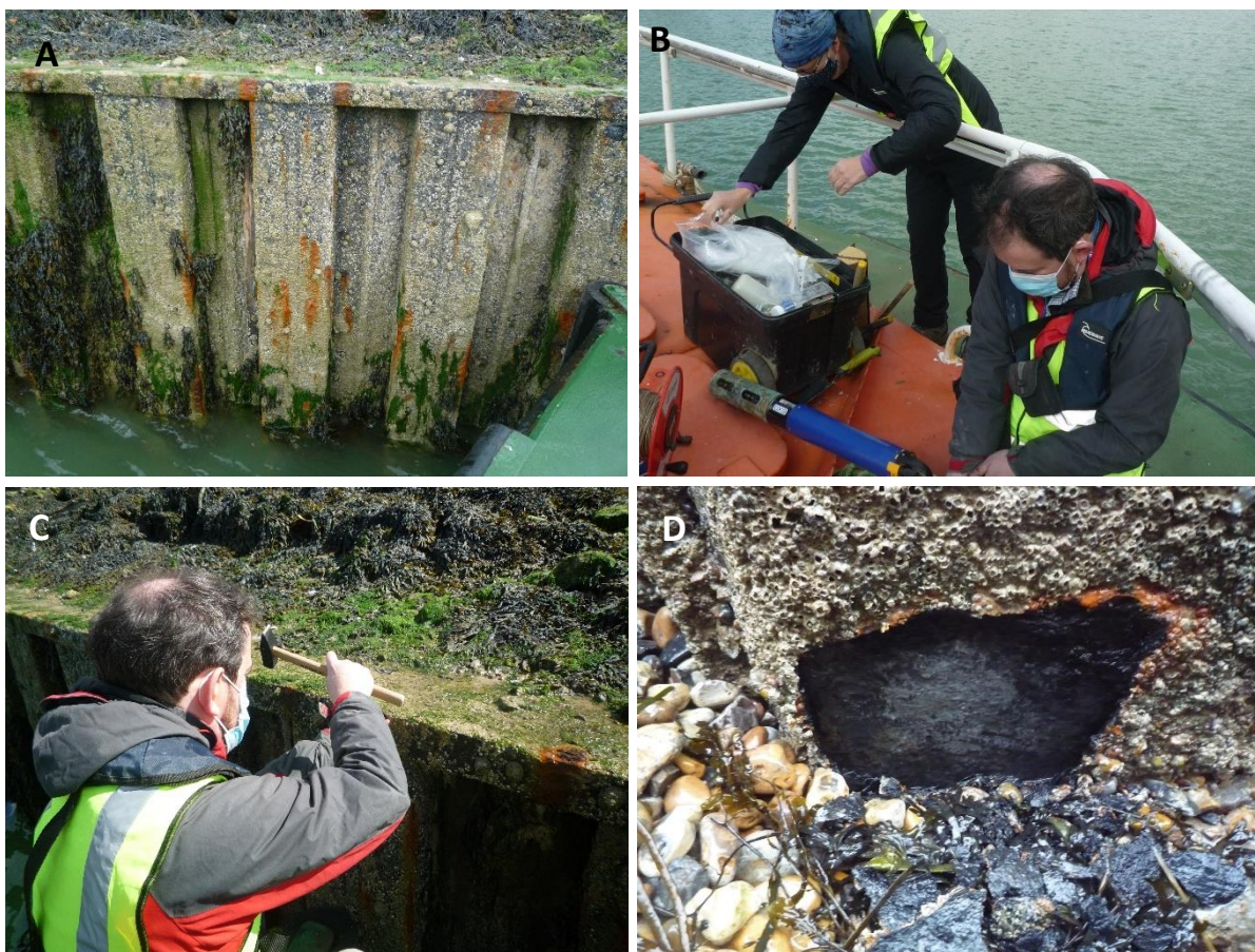
Figure NH2: Images of Newhaven Port environment and corrosion. (A) View of the steel pile wall. (B) Water and corrosion sampling from pilot boat. (C) Corrosion sampling from pilot boat. (D) Removed intertidal corrosion blisters show inner sulphidic layer and acid etched steel.
