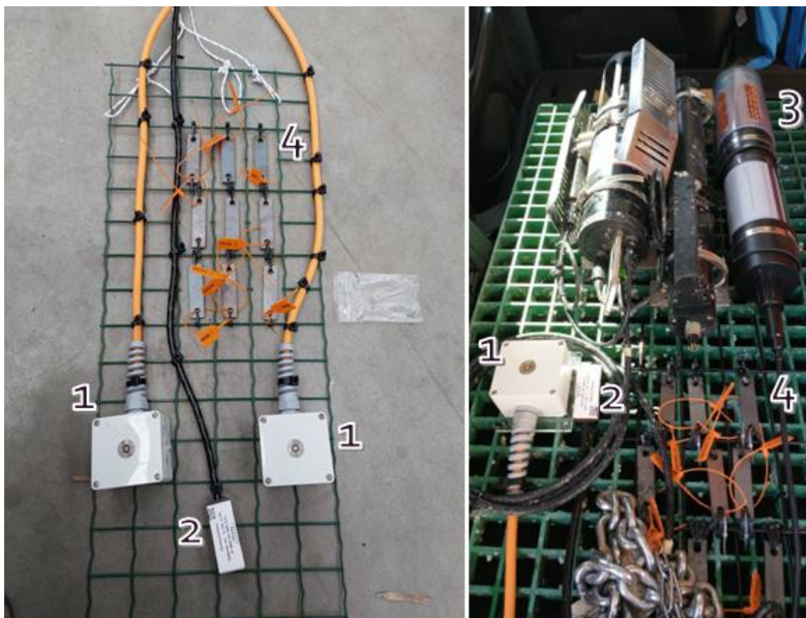
Figure 8: Left: Frame with corrosion coupons and sensors for installation on the inside of the MP. Right: Sensors and corrosion coupons installed on the outside of the MP. (1) C-Cube sensors, (2) COSASCO sensors, (3) Manta Multisensory probes and (4) corrosion coupons.
