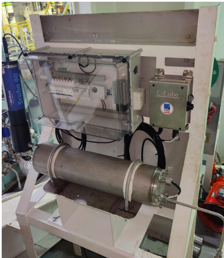
Figure 32: Electrical cabinet ballast water sensor system and C-Cube controller.
