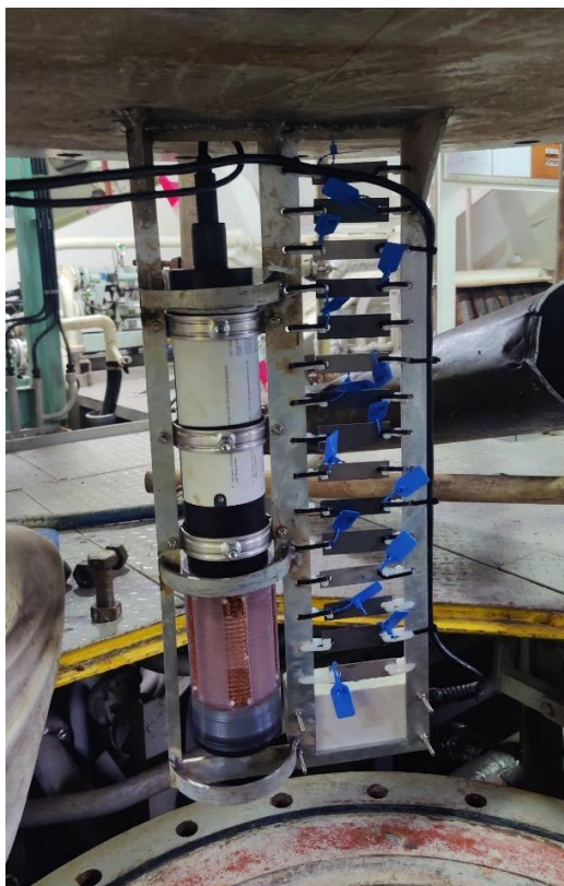
Figure 14: Sensor rack with Scuba sensor, C-Cube sensor and corrosion coupons, lifted out of the strainer.
