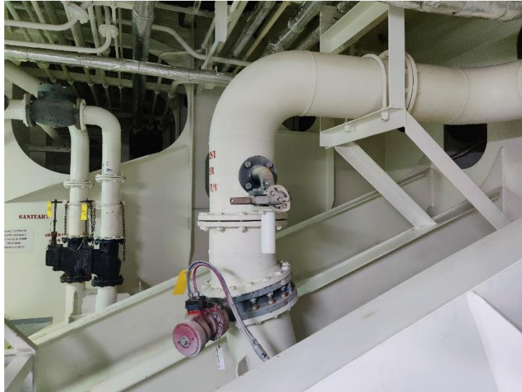
Figure 20: Ballast water discharge line
