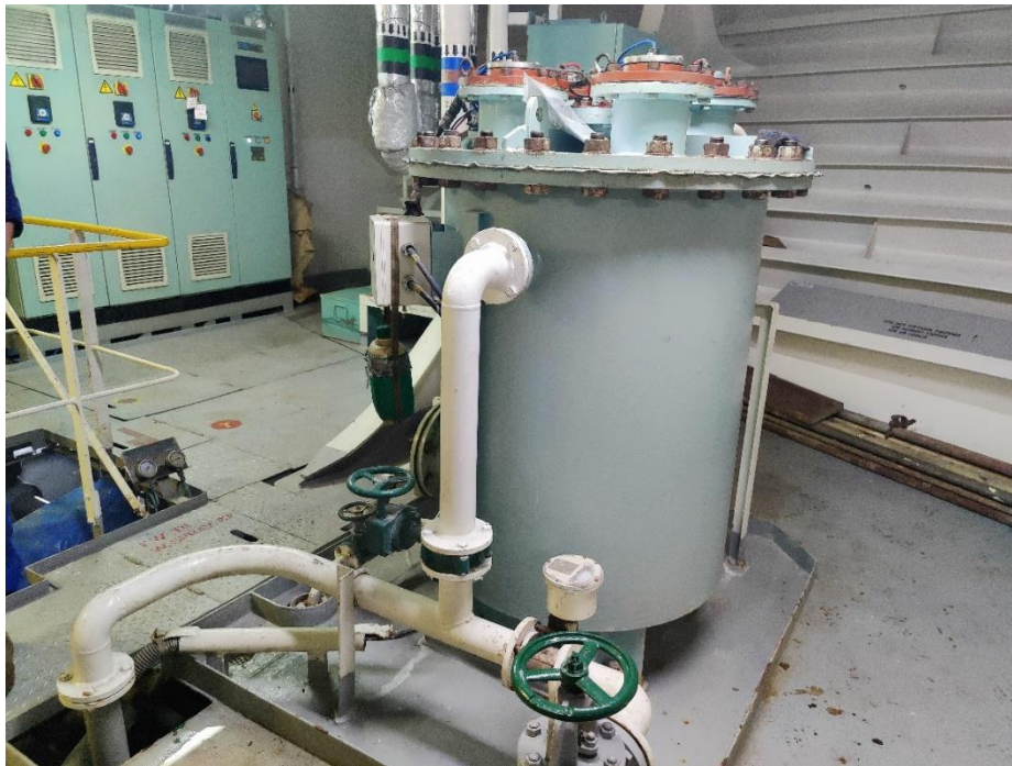
Figure 12: Antifouling (MGPS) anode treatment tank
