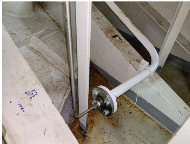
Figure 28: Reducer in the supply line for the flow cell.
