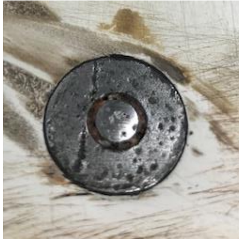
Figure: Local corrosion attack (pits) on the S355 working electrode of the C-Cube LPR probe after 6 months of installation in the MBBR installation – Putte (Greenhouse)
