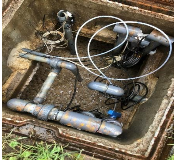
Figure 1: The MBBR with the installed C-Cube and Manta probe
