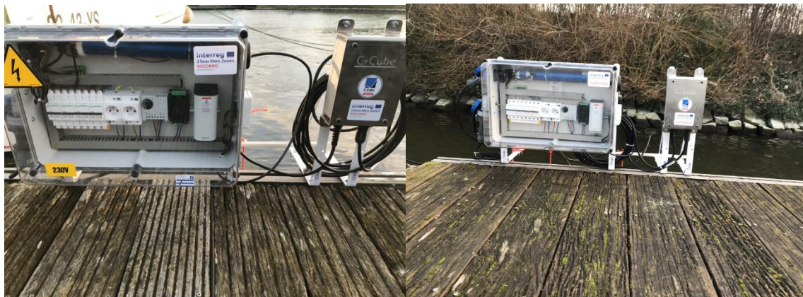
Figure 2. Sensor box on the north side (left) and the south side (right) of the Zelzate marina
